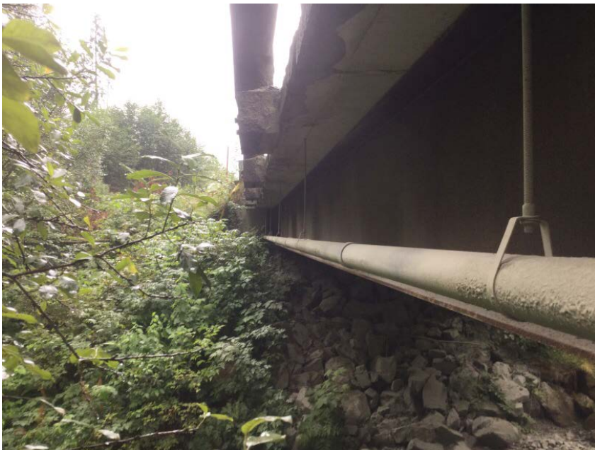
Utilities hung from deck
