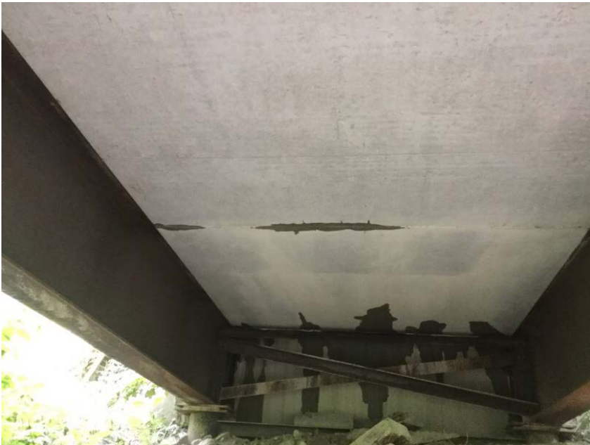
Water getting through deck joints but not severe
